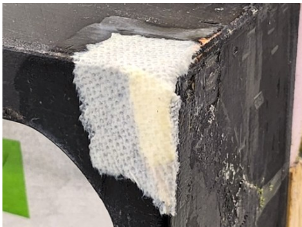
(Pic 10) A different corner with a missing section. The missing piece was repaired (yellow portion) and the next day we applied the outer patch, ready for the final glue application.
