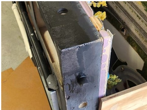
(Pic 9) The last step for the repairs is a light sanding and painting to seal the patch from any moisture.
