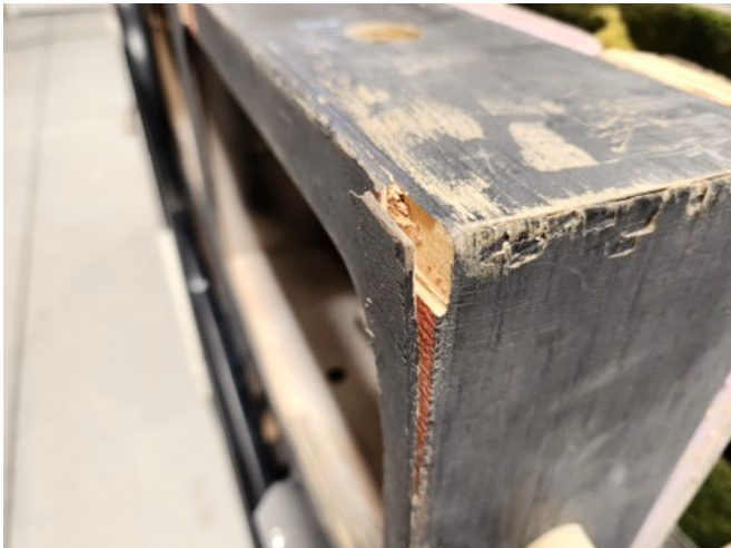
(Pic 7) This corner took a big hit with the plywood delaminated for several inches. First wood glue was applied to the inside of the delaminated section and was clamped overnight. The repair patch was applied the next day.
