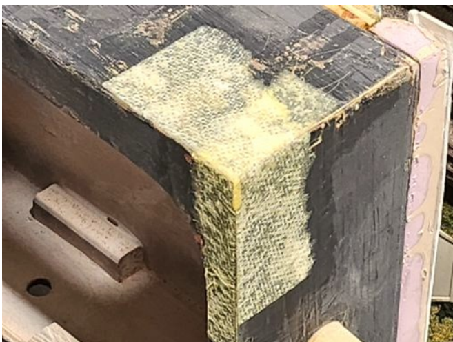
(Pic 8) The same corner after the Fiberpaper patch was applied and dried.
